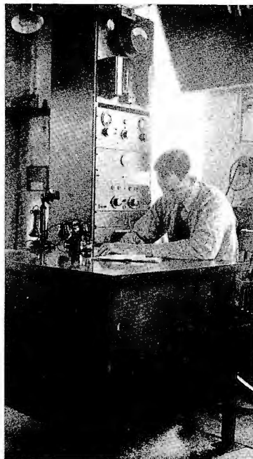
A corner of the control room.
